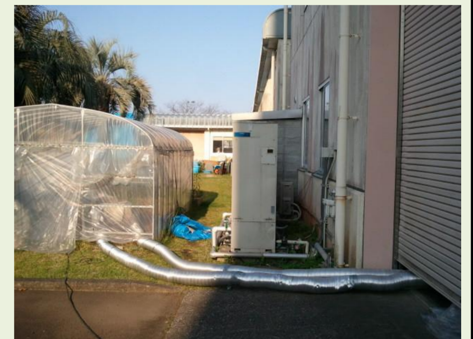
Green house air-conditioning
